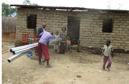
Zamda's house covered with borrowed torn out metallic sheets. Nininahazwe provides new metallic sheets to cover the roof
